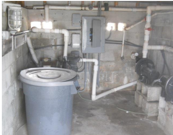
INTERIOR VIEW: PUMP HOUSE
